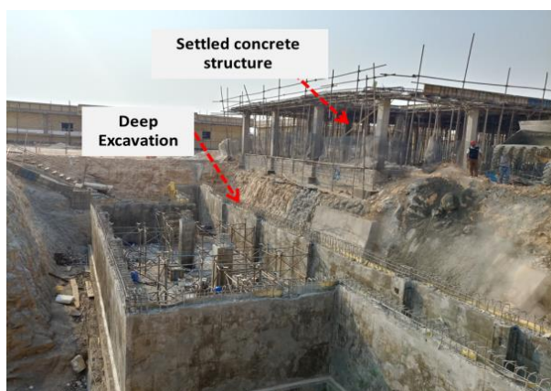
Fig. 1. The concrete construction near the excavation has suffered subsidence
